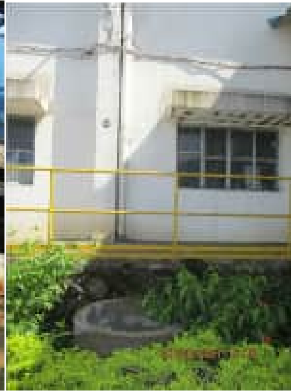
2. Rainwater recharge pit of Building roof
